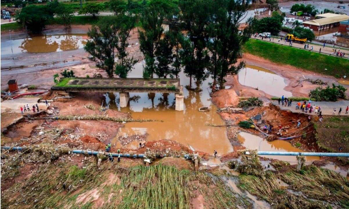
This picture shows damages from floods, in South Africa, which occurred in April 2022 – in KwaZulu-Natal Province.
